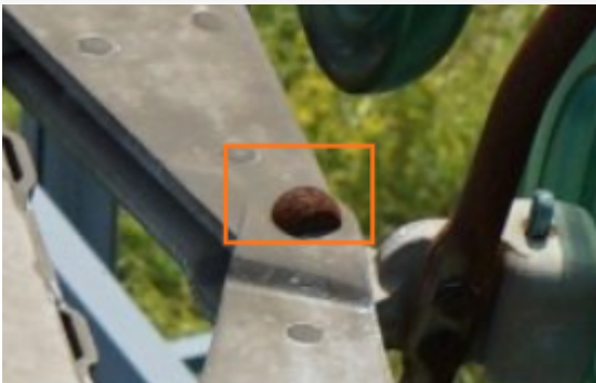
882892 Severity: 2 rust on bolt
