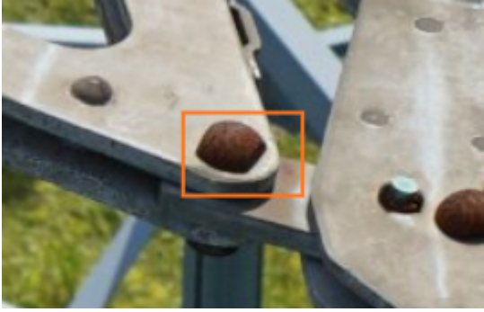
882895 Severity: 2 rust on bolt
