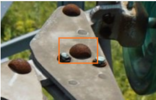
882891 Severity: 2 rust on bolt
