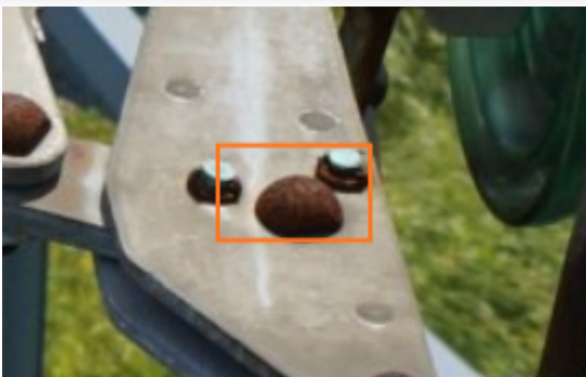
882893 Severity: 2 rust on bolt
