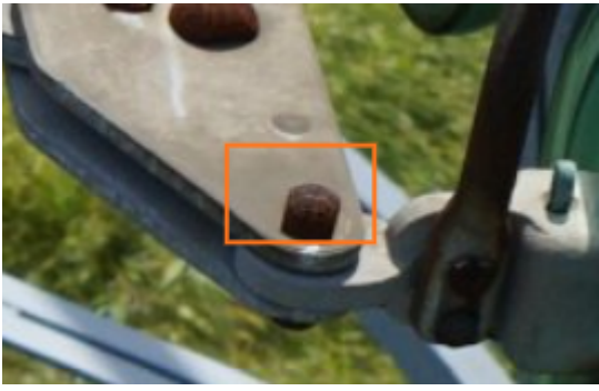
882894 Severity: 2 rust on bolt
