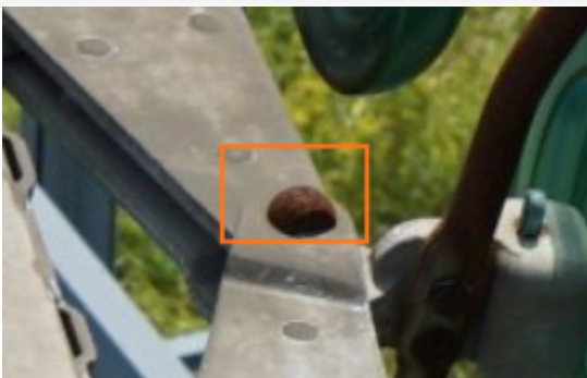
489856 Severity: 2 rust on bolt
