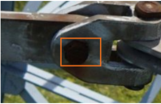
489853 Severity: 2 rust on bolt
