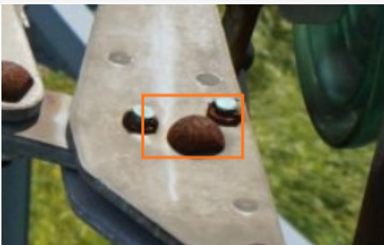
489857 Severity: 2 rust on bolt
